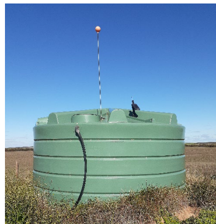
Remote tank monitoring
