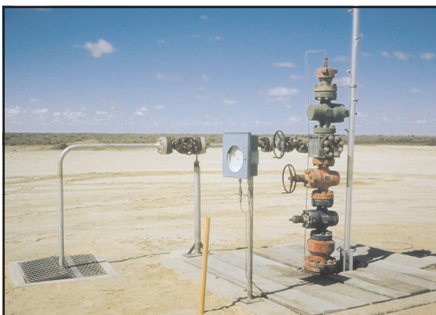
Well head of a Tirrawarra Field gas injector. (Photo 35486)
