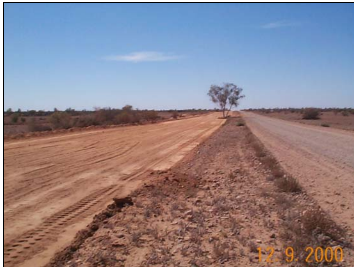
Plate 2: Clear and grade of a reduced-width right-of-way adjacent to an existing track
