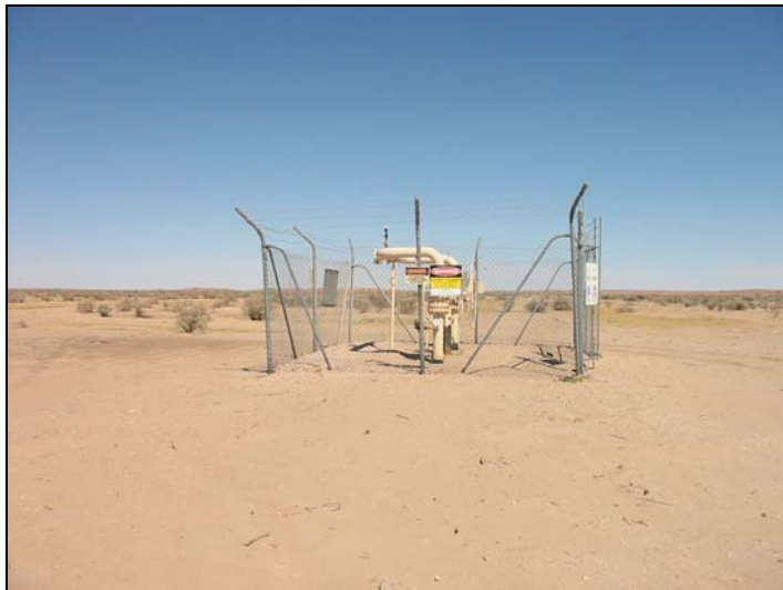
Plate 1: A Mainline Valve compound
