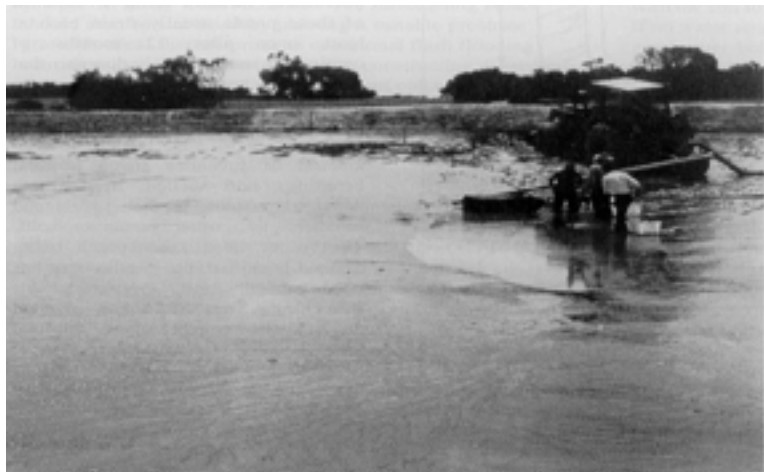
Pond almost completely drained. Note that the bottom in this pond was firm enough to follow the falling water level into the sump by tractor with the pump attached.
