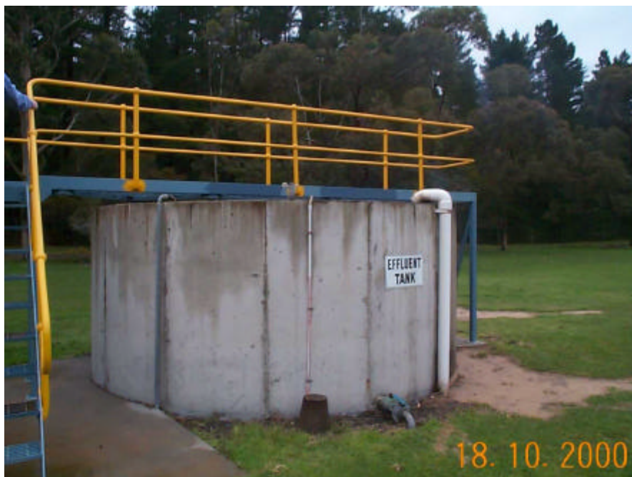
Plate 5: "Effluent" storage tank.
